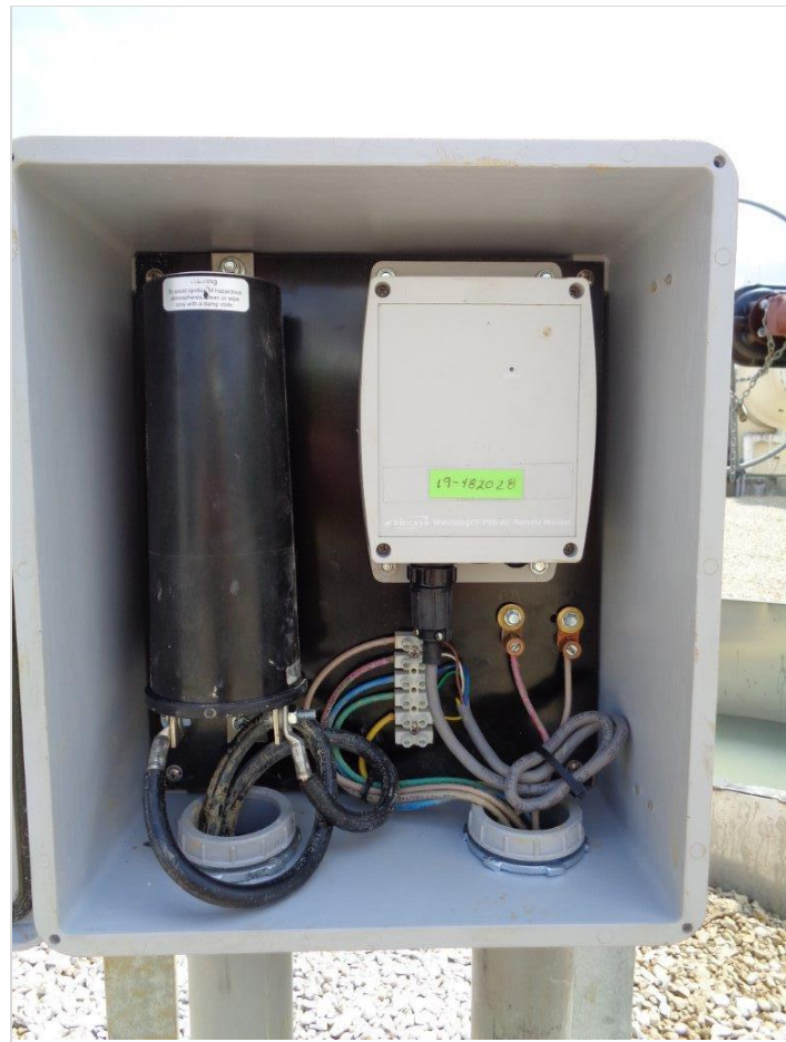
Figure 1 – Junction box with solid state decoupling device and monitoring unit
