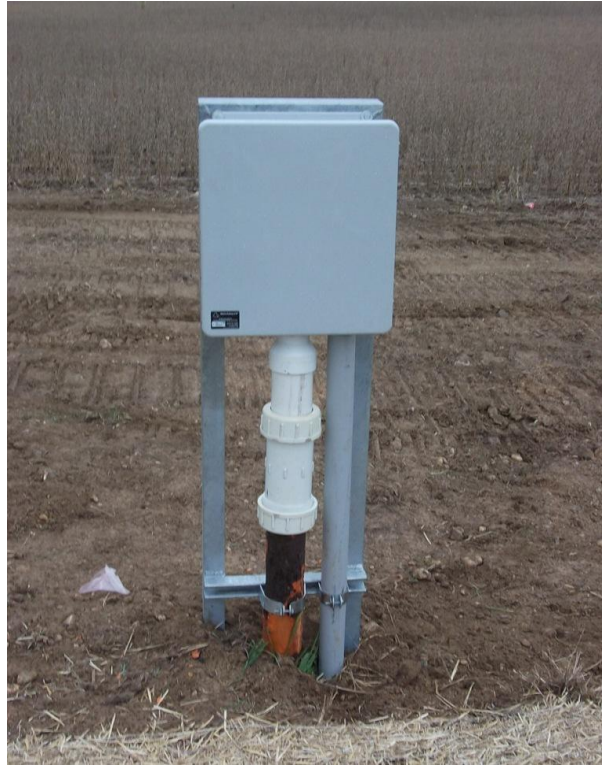
Figure 7: Photo of monitor equipment installed.
