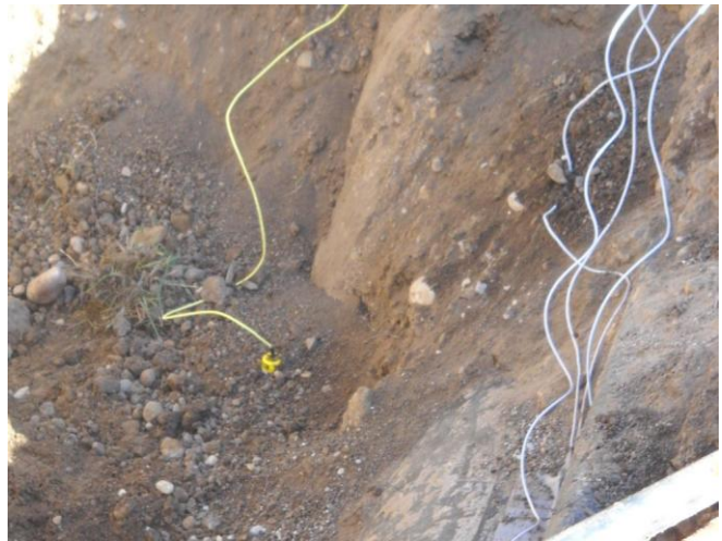
Figure 6: Installing the reference cell.
