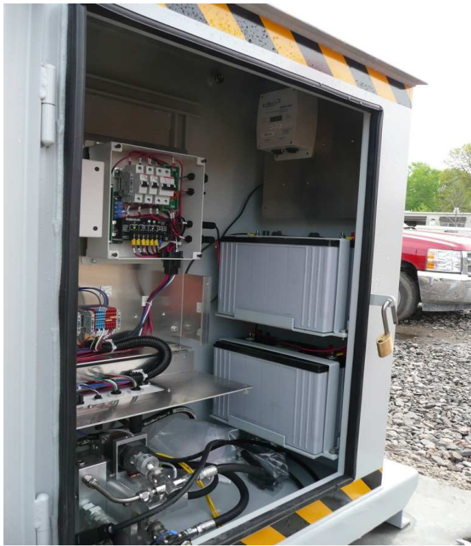
Figure 9: Monitor Inside TOR unit
