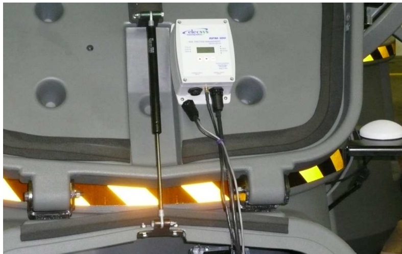
Figure 13: Close Up of Monitor Inside GF Unit
