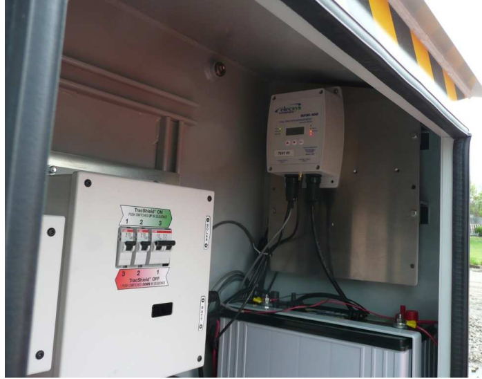
Figure 10: Monitor Inside TOR Unit
