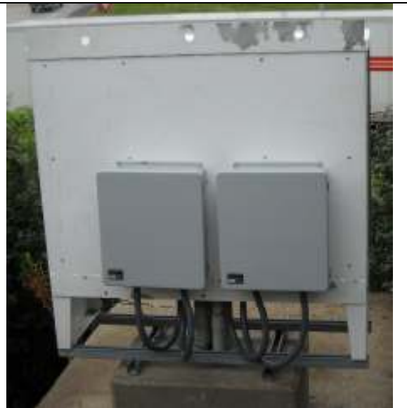
Figure 10: Two 3-Zone enclosures mounted at a six zone rectifier site.
