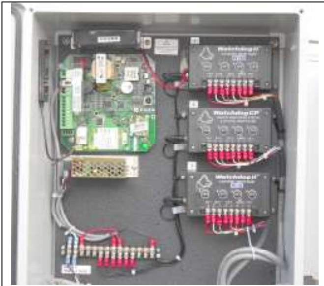
Figure 9: Interior view of a 3-Zone integrated enclosure.
