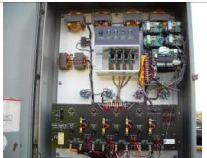
Figure 2: Photo of rectifier enclosure with monitor system installed in upper right side.
