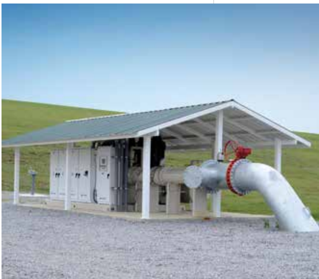
Watertronics customized pump station at Dee River Ranch.
