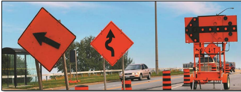
Work zone signage and delineation can create confusion and allow intrusions
