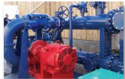
Horizontal pump station
