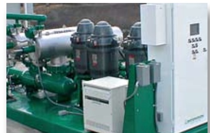
Vertical pump station
